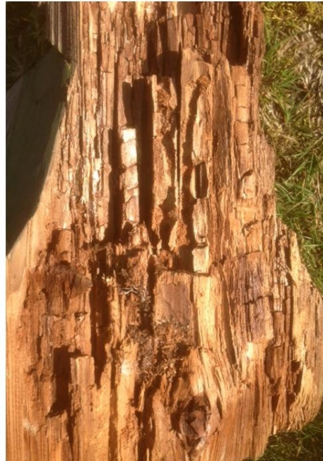
FIG 2—Advanced decay in top feature
