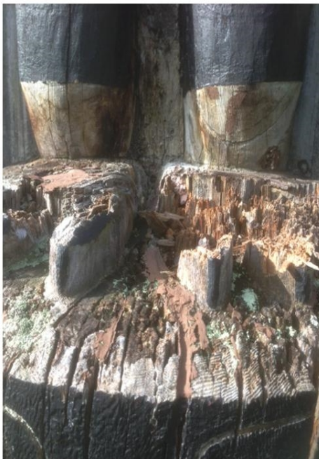
FIG 3—Decay in lower section
