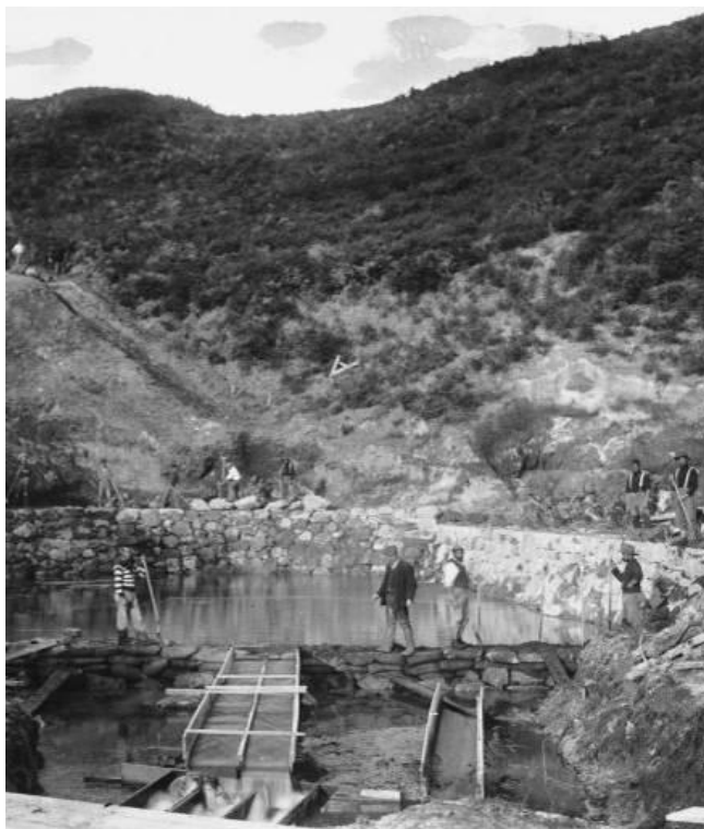
The reservoir at Rotorua under construction c 1910 P A Coll 6075-54, Alexander Turnbull Library, Wellington.
