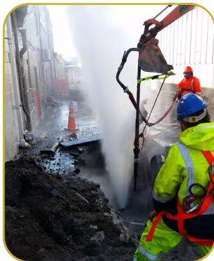
Figure 3 Bore Failure, 2016 (photo: Andrew Austin).
