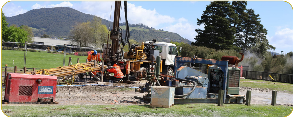
Figure 21 Example of space required around a bore for a drilling rig and plant (photo: Rotorua Well Drillers).
