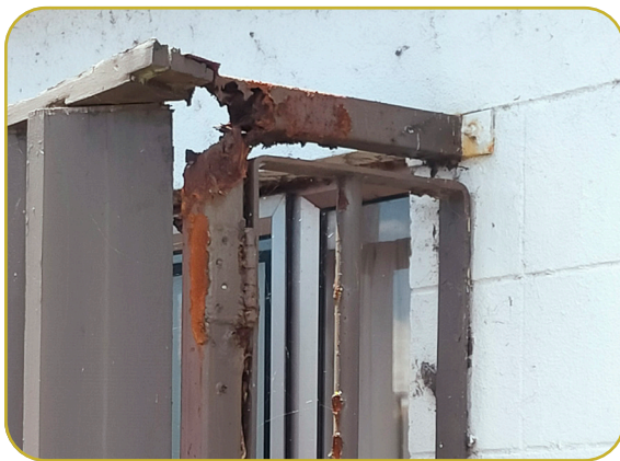
Figure 7 Accelerated corrosion on a building near Sulphur Bay (Photo: Kim Smith, January 2024).
