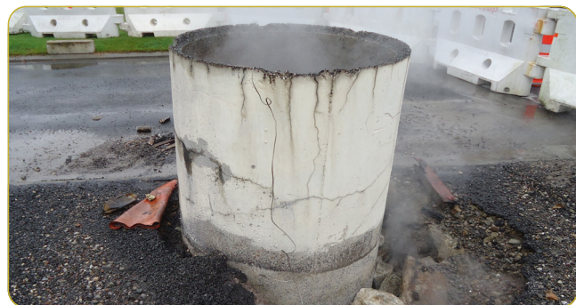
Figure 4 Bore Casing Failure (photo: Rotorua Lakes Council).
