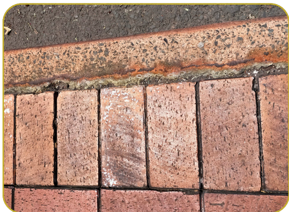
Figure 15 Concrete edging at ground level affected by geothermal conditions (photo: Kim Smith, January 2024).
