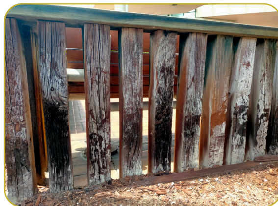
Figure 16 Timber affected by geothermal conditions (photo: (Kim Smith, January 2024).
