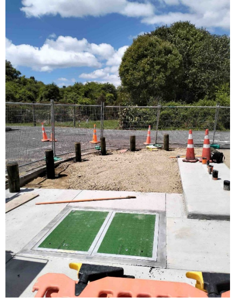
Transfer Station Pump Station
