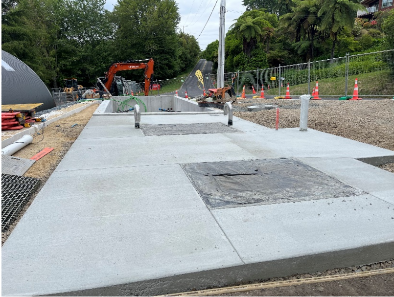
Stoney Point Pump Station
