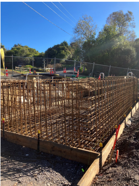
Cliff Road Pump Station
